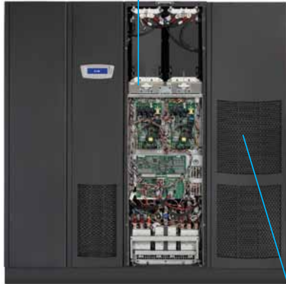
Concurrent maintenance in Eaton 9395 550 kVA
